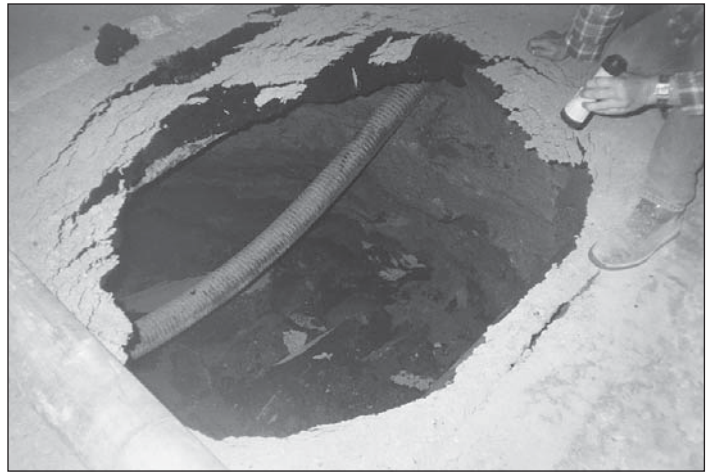
Subsidence pit, about 6 feet across and 8 to 10 feet deep, on I-70 resulting from roof collapse of a mine in March 1995. Photo courtesy of Gannett Fleming, Inc.
