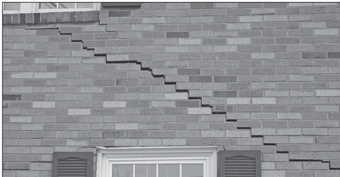
This home in Sugarcreek, Tuscarawas County, was damaged by the collapse of an underground mine. July 9, 2009.
